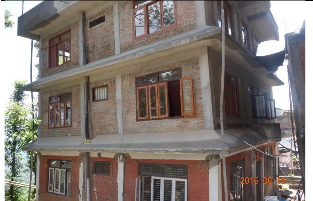
Fig. 4.4 Building with multiple column failure
